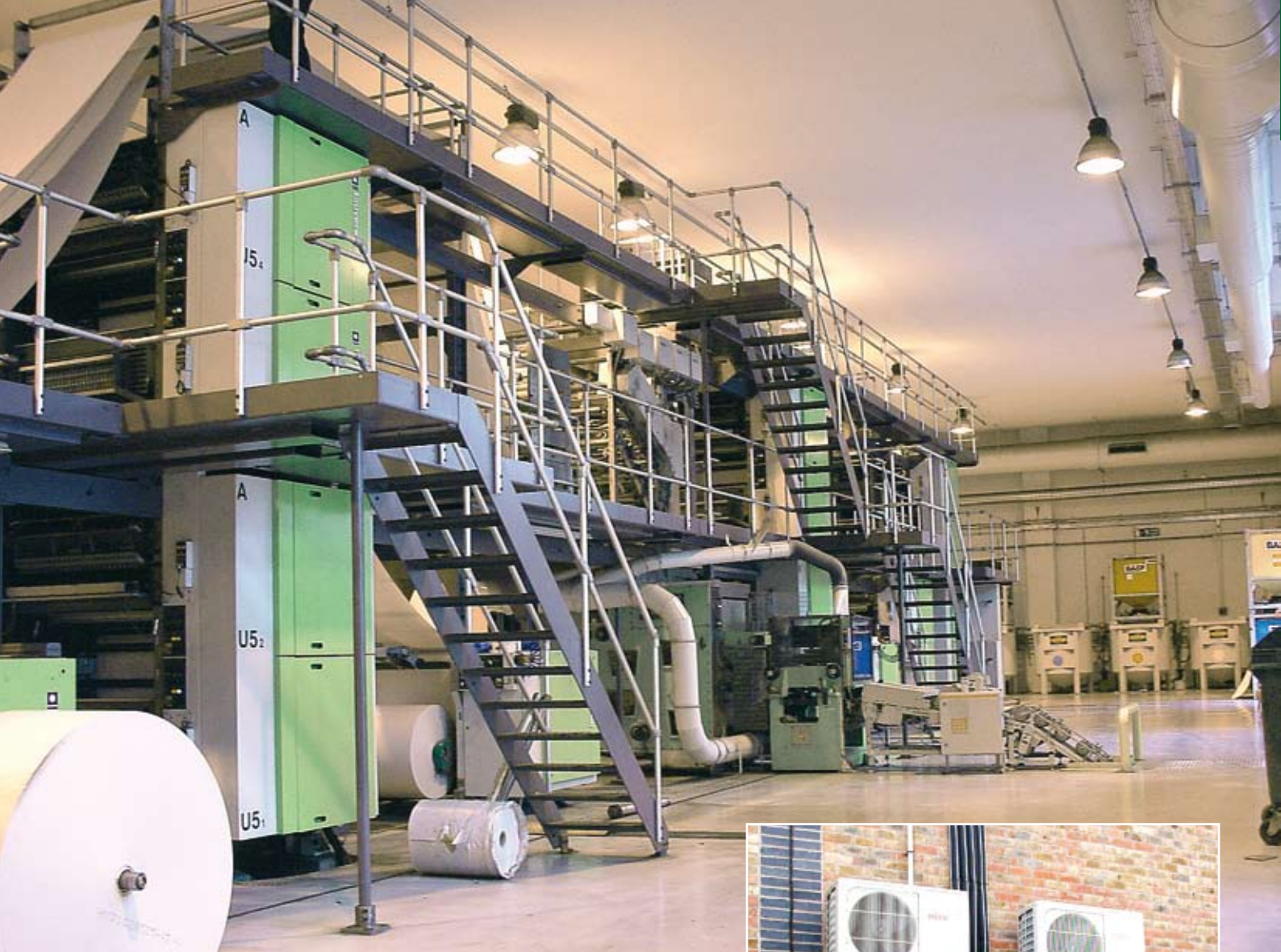
The machine room at Friday Ad's Sayers Common headquarters, and (right) the Fujitsu condensor units.
