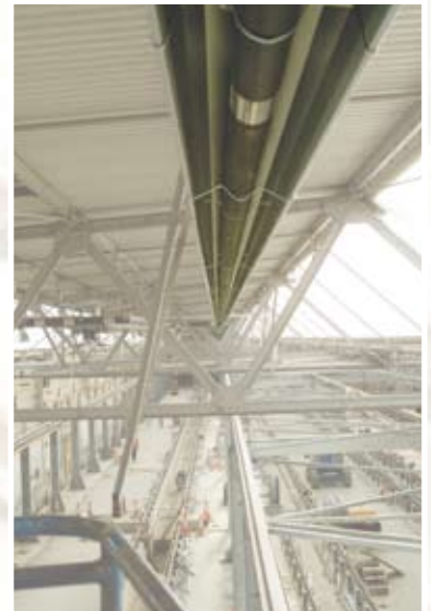
Below: The business end of the Ambi-Rad Nor-Ray-Vac system installed at Brighton
